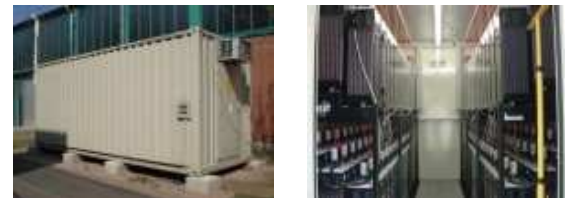
Figure 3: Battery storage with system voltage of 384 V consisting of 192 single cells.
